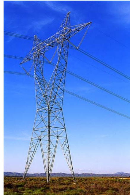
Transmission Facilities: Higher-voltage
